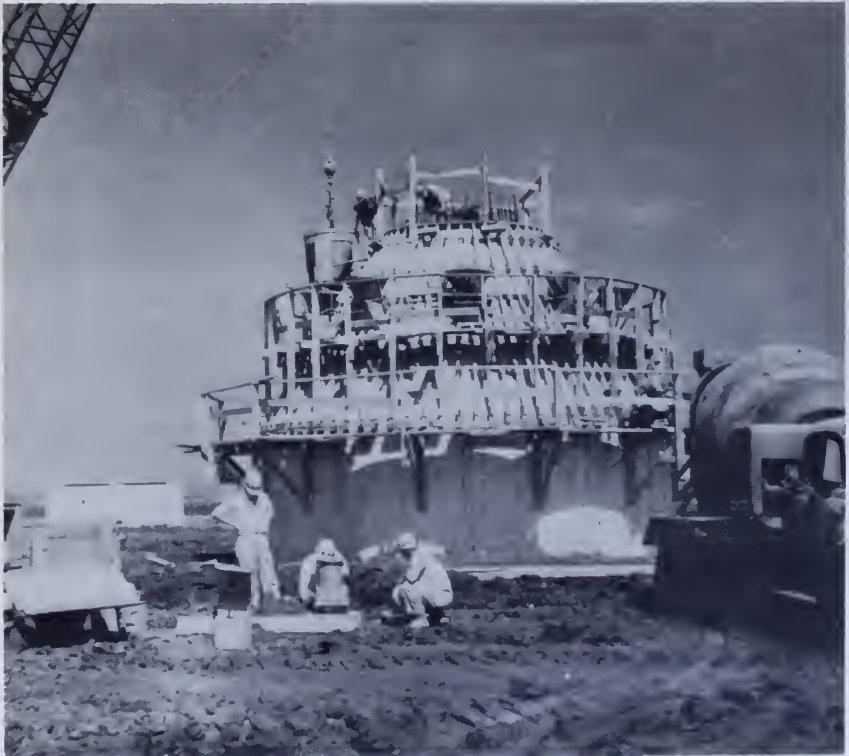
Figure 62.—A concrete platform provides a stable test area on the Wichita project. P835-526-682.
